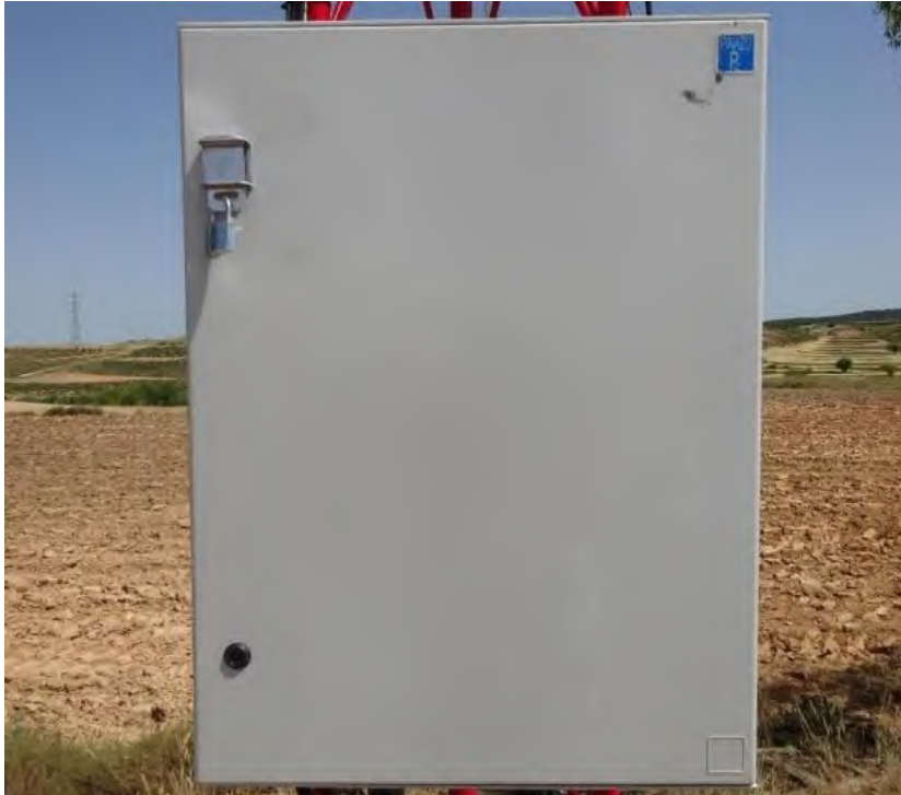
Exterior of cabinet
