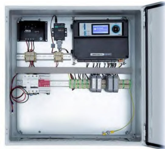
Cabinet with data logger and communication system
