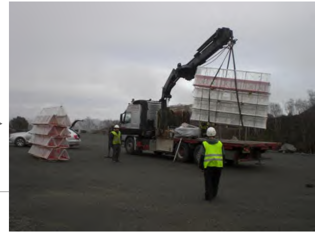
3. Met masts will be offload with a small truck of minimum 5m from the containers to the warehouse
