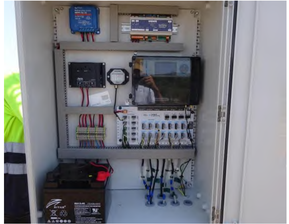
Interior of cabinet
